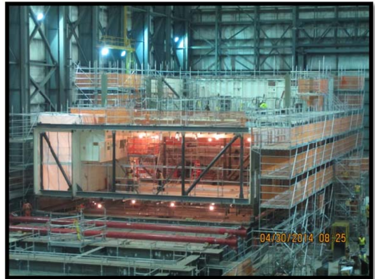
Inside Topsides module hall - April 2014
