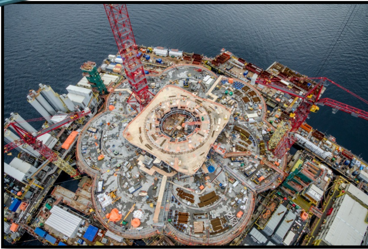
Gravity Based Structure (GBS) girder star formwork in place for the centre shaft slip form pour
